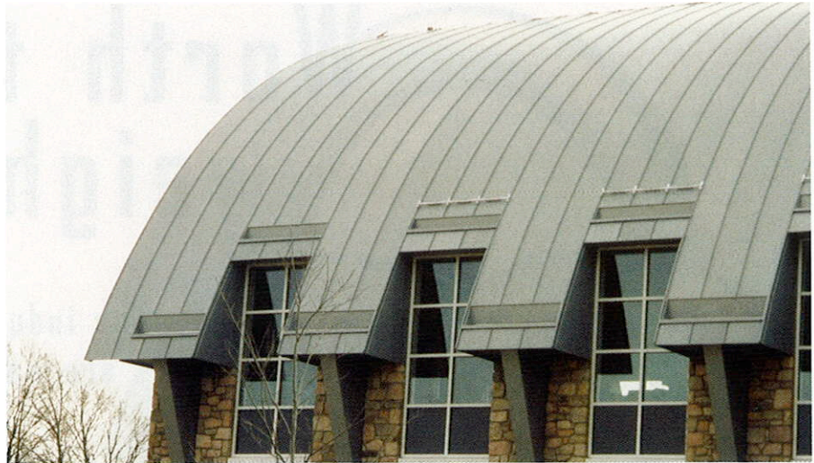
Gooding Simpson & Mackes Inc., Ephrata, Pa., installed a RHEINZINK Metal roof system on the Lititz Watch Technicum.
